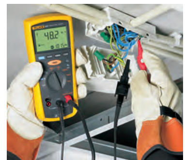
Wiring Test in a small Distribution Box – all in one Spot
